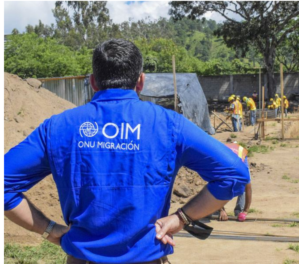
Nicola Graviano, IOM Chief of Mission in El Salvador and Honduras visiting the shelter's construction site for migrants in transit. IOM 2023 / Ismael Cruceta. © IOM 2023
